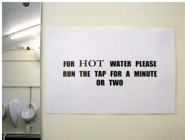
Figure 8. Energy and water wastage due to dead legs is difficult to quantify but a daily experience.
