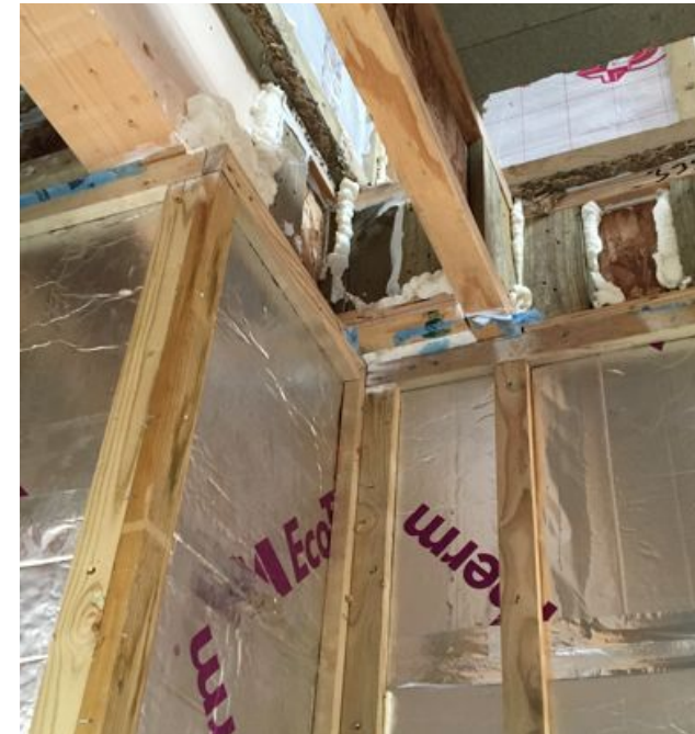
Necessary remedial work took undertaken by inexperienced people
