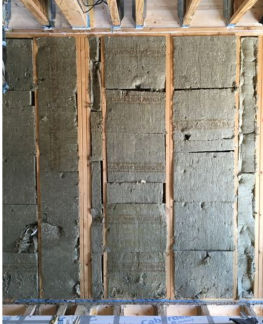
No quality checks undertaken during construction
