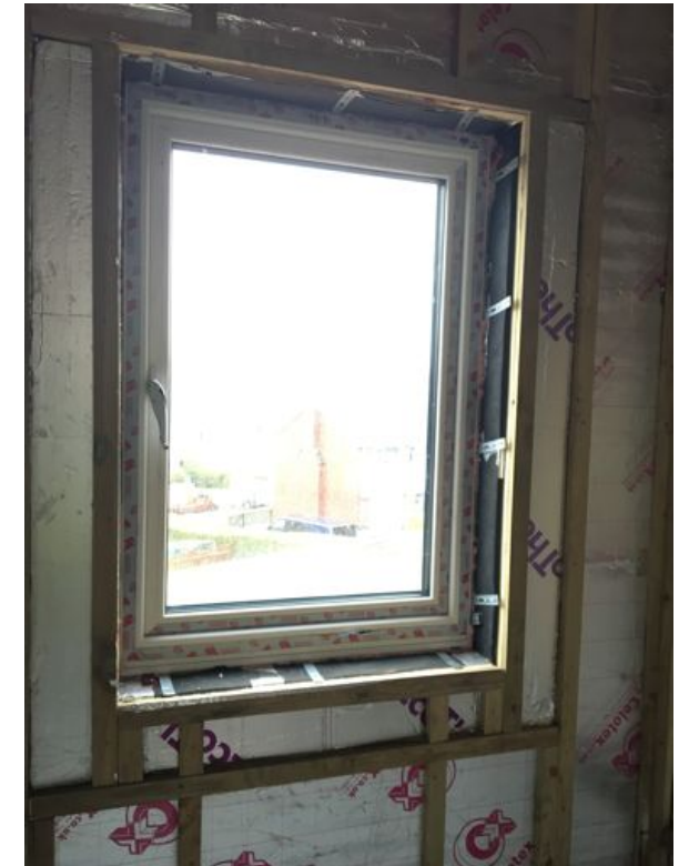
Airtightness designed in inaccessible place once closed off
