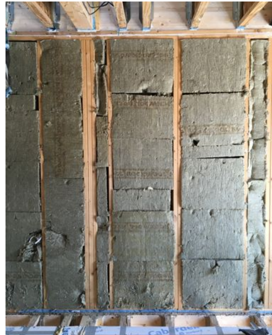
No quality checks undertaken during construction
