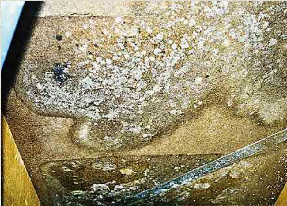
Fig.: Moisture damage and mould growth at the subroof (timber fiber board)
