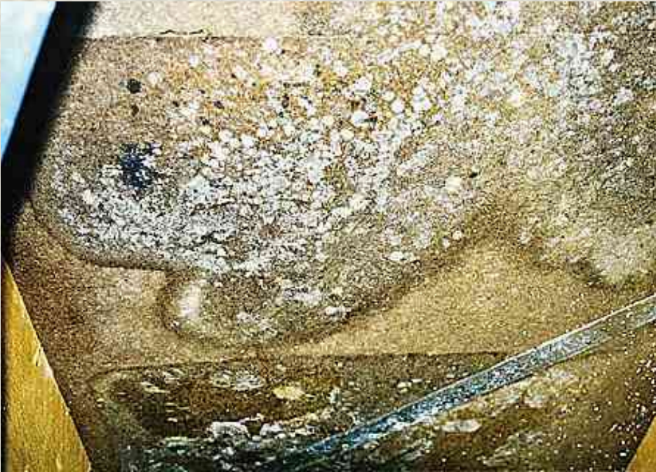
Fig.: Moisture damage and mould growth at the subroof (timber fiber board)
