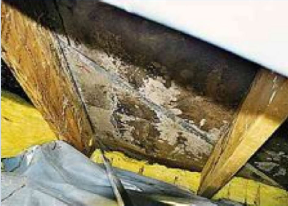
Fig.: Moisture damage and mould growth on the subroof
