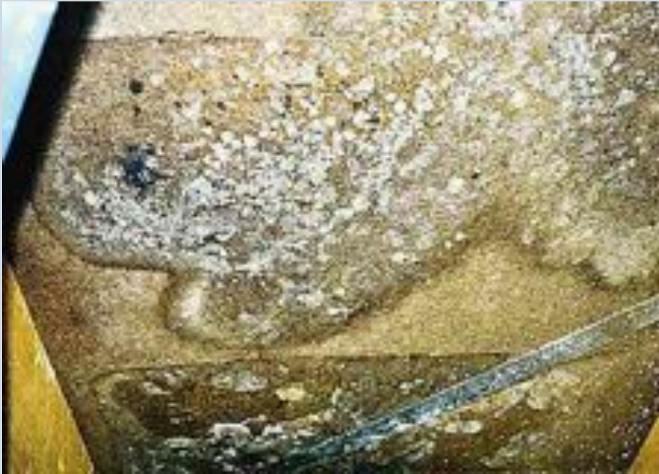
Fig.: Moisture damage and mould growth at the subroof (timber fiber board)
