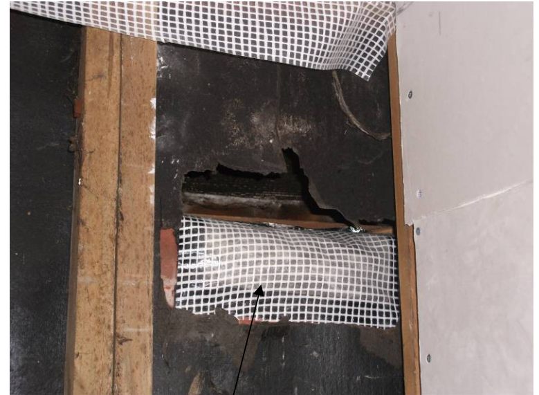
Original air grate filled with insulation & sealed with VCL & made air tight.
