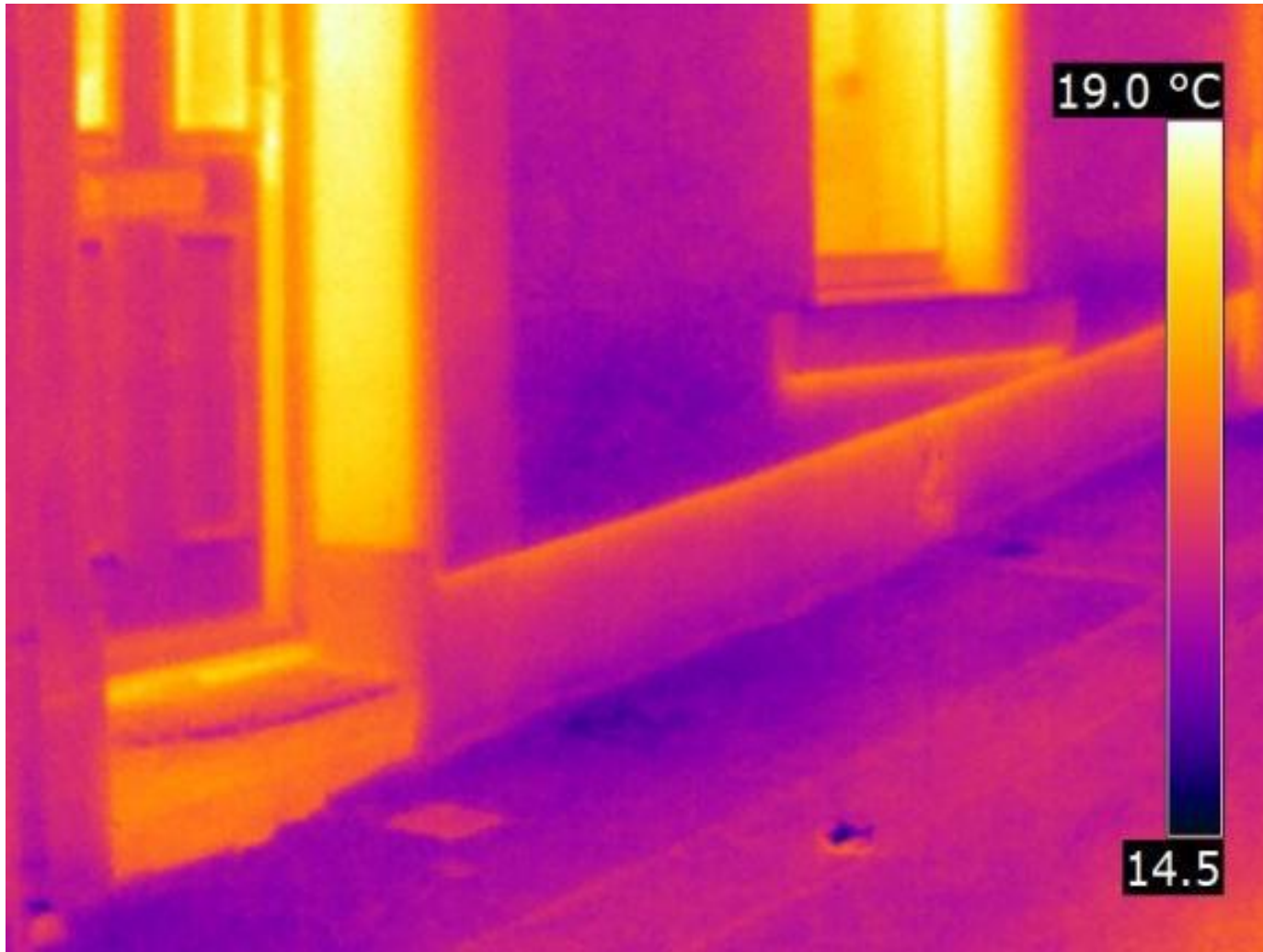
Assessing the execution of retrofitted external wall insulation for pre-1919 dwellings in Swansea (UK); Joanne Hopper et al 2011
