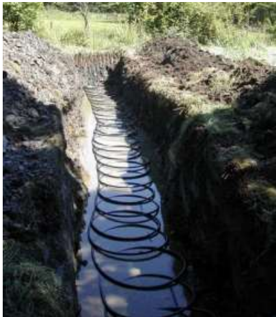
Ground source heat pump £11,000
