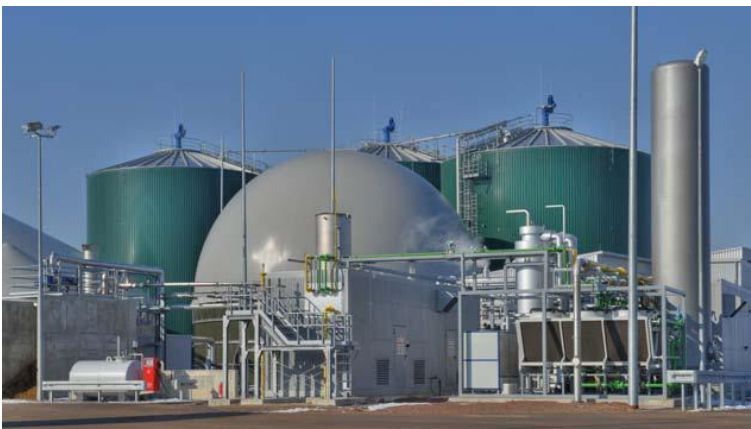
Figure 19. A 7 MW anaerobic digester at Güterglück, Germany. 215 Courtesy: RWE.
